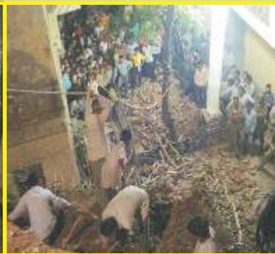
Inflatable light Tower for Relief and Rescue Operations at building Collapsed site
